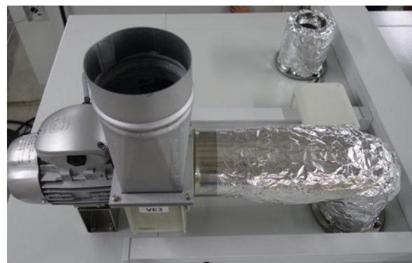
FLUSHING / PRESSURE RELIEF SAFETY
